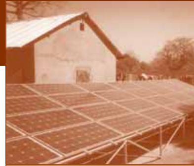
Autonoom PV-systeem in Gambia (Solar Technics)
